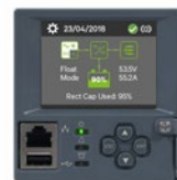
Individual current measurement for each fuse/breaker
